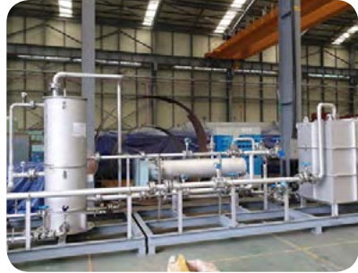
Glycol Water Heating System
